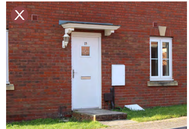
Visually intrusive metre boxes onto street
