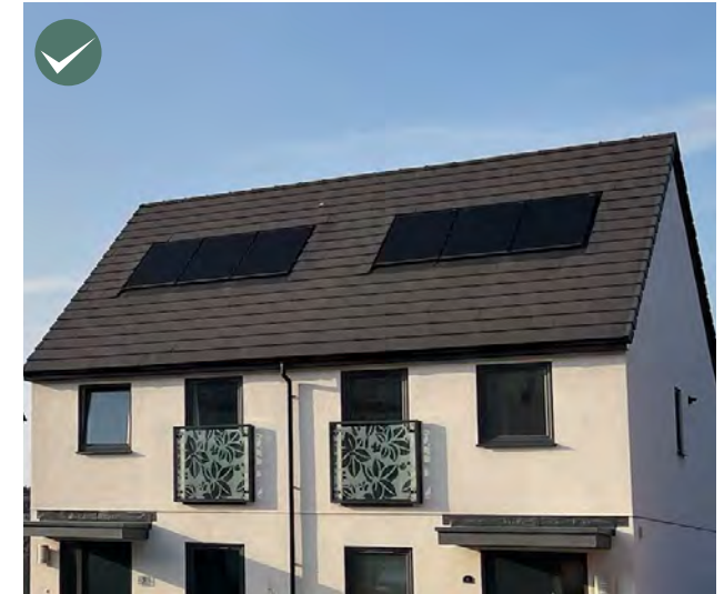
Solar PV arrangement uniform and centred
